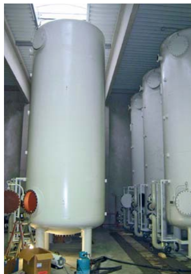
New machinery and equipment are being installed at the leather factory in Feldbach to assure more efficient effluent cleaning.
